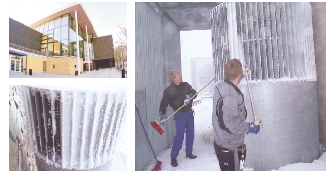
FIGURE 6. De-icing the air intake for a school building in Trondheim, Norway. The school was built in 2004 and the photos taken in early January 2006. Photo: Fredrik Hedeman.
