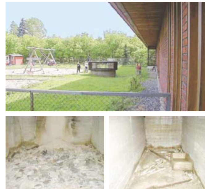
FIGURE 19. Air intakes at easily accessible heights can become waste bins. Abandoned building waste does not improve the situation. Photo: Frode Frydenlund, EPT-SEfAS.
