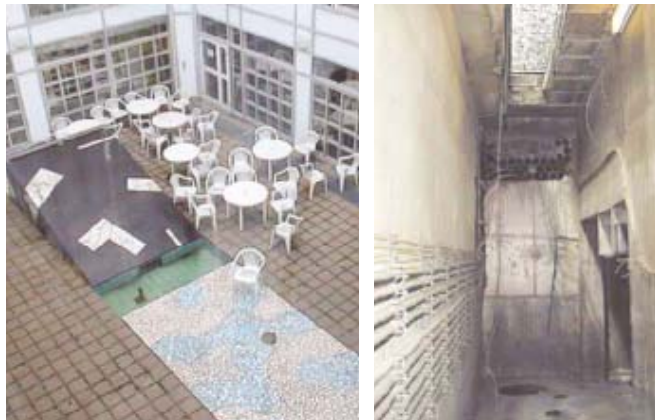
FIGURE 20. Intake grilles located at ground level. The open space is often used by smokers and the grille is partially blocked by cigarette ends and other debris. Photo: Frode Frydenlund, EPT-SEfAS.
