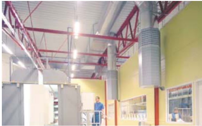
FIGURE 45. Displacement diffusers with both horizontally and vertically oriented spread patterns.
