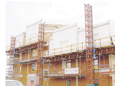
FIGURE 4. Requirements for achieving a good indoor environment can include the provision of weather and moisture protection measures for materials and components, to protect them against moisture and dirt.
