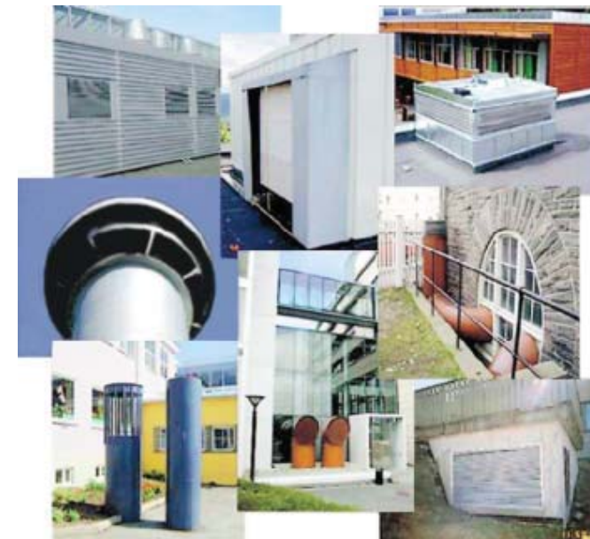
FIGURE 1. Different types of air intakes for public and commercial buildings. Some of the intakes have not been designed or located according to Norwegian regulations and recommendations. Those shown bottom-right are substandard in all respects.
