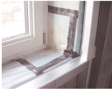
FIGURE 5. An airtight building envelope is another important requirement for good air quality and energy efficiency. There is sometimes a misunderstanding about whether or not leakage and infiltration through the building envelope is beneficial. A building must, of course, be allowed to breathe but this is a job for the ventilation system.
