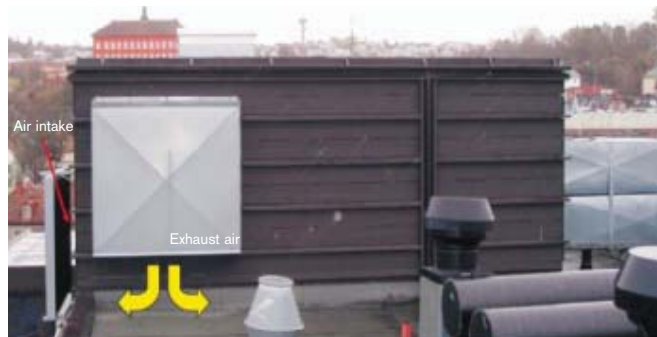
FIGURE 7. Unsuitable location of an outdoor air intake in relation to the exhaust air outlet. There is a great danger of short-circuiting between the two systems and undesirable microbial growth on the surface of the roof – microbes could then find their way into the air intake. Photo: Frode Frydenlund, SINTEF Energy Research, 2007, Trondheim, Norway.
