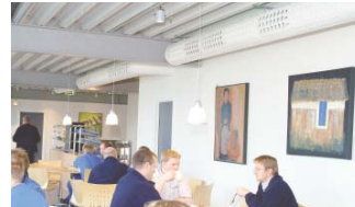
FIGURE 30. Duct diffuser installed in a restaurant.
